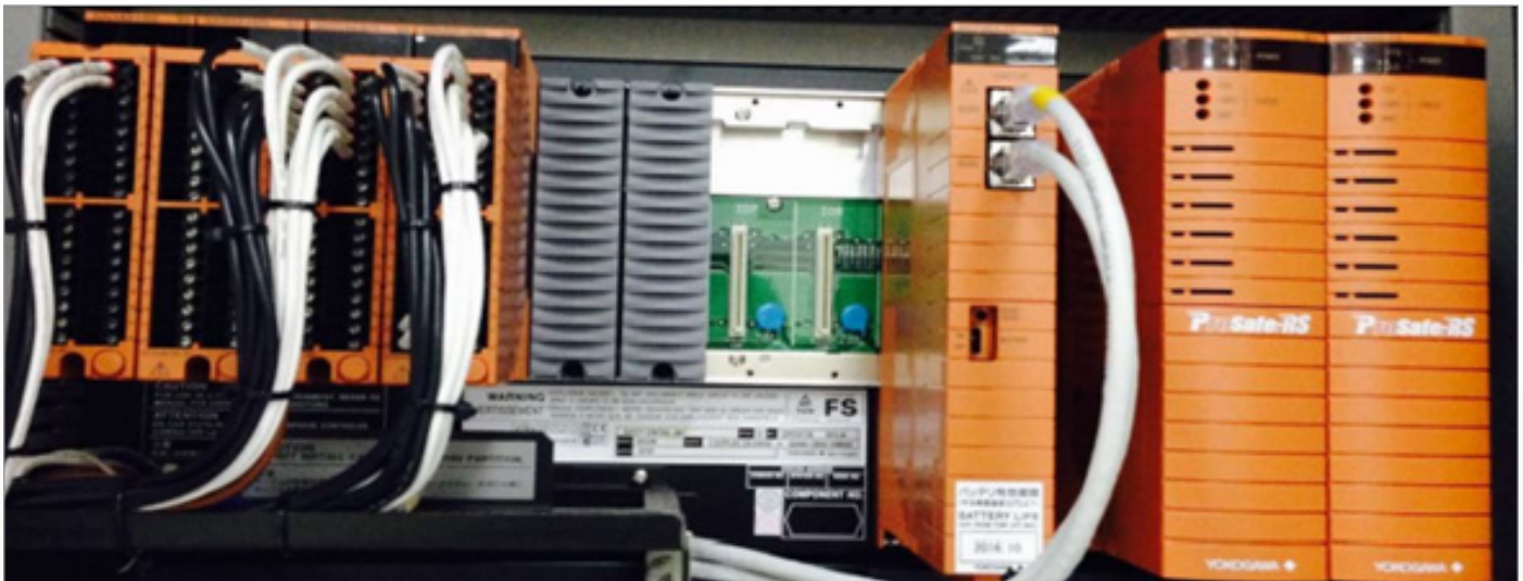
Fig.1: 1- redundant power supplies 2- Central processing Unit (CPU) 3- Analog input module 4- Analog output module 5- Digital input module 6- Digital output module
