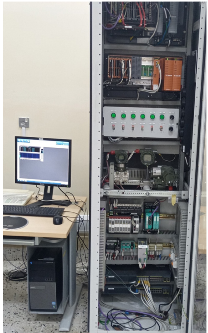
Fig.1 DCS system at UOB: 1-Field Control Station (FCS) 2- Emergency shut down (ESD) 3- Engineering
